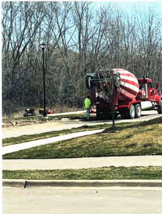
Ozynga Concrete washing their truck shoot directly into the curbside inlet. This is adjacent to what the SWPPP listed as a protected wetland
