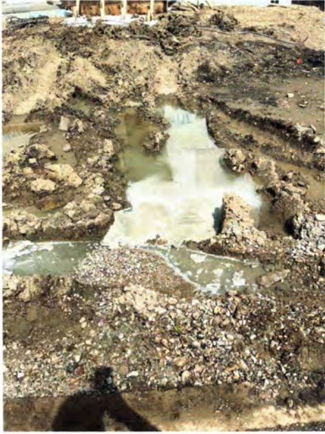
Concrete washout in tire tracks where the concrete trucks were entering the site via the ramp.
